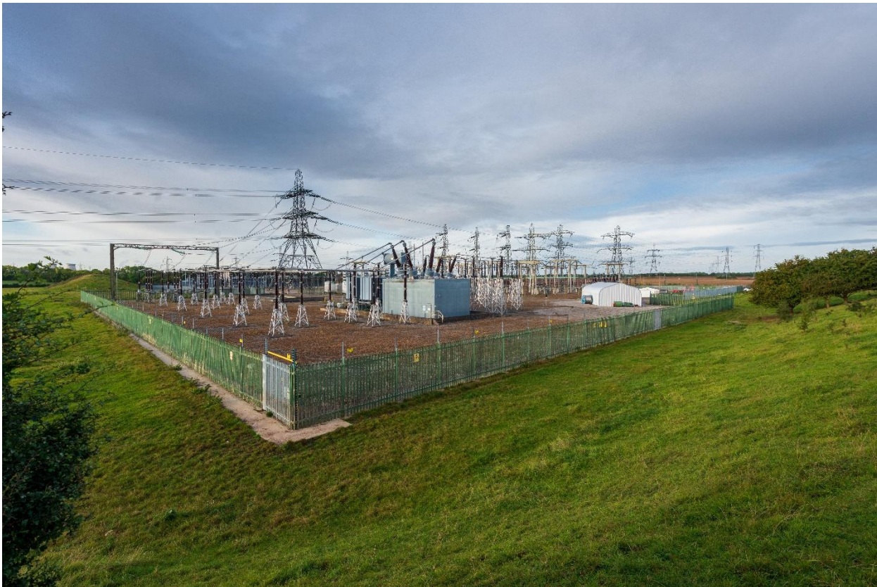
Figure 4.2 – Typical substation (existing Monk Fryston Substation)
