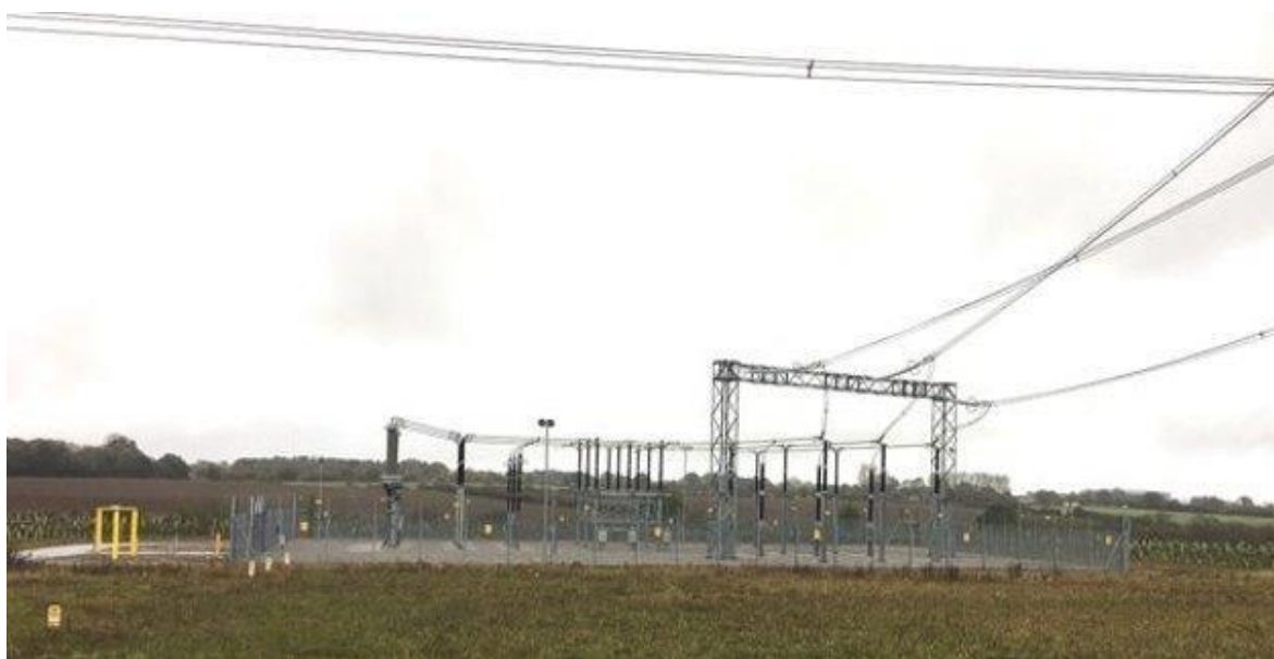
Figure 4.1 – Example of Cable Sealing End Compound
